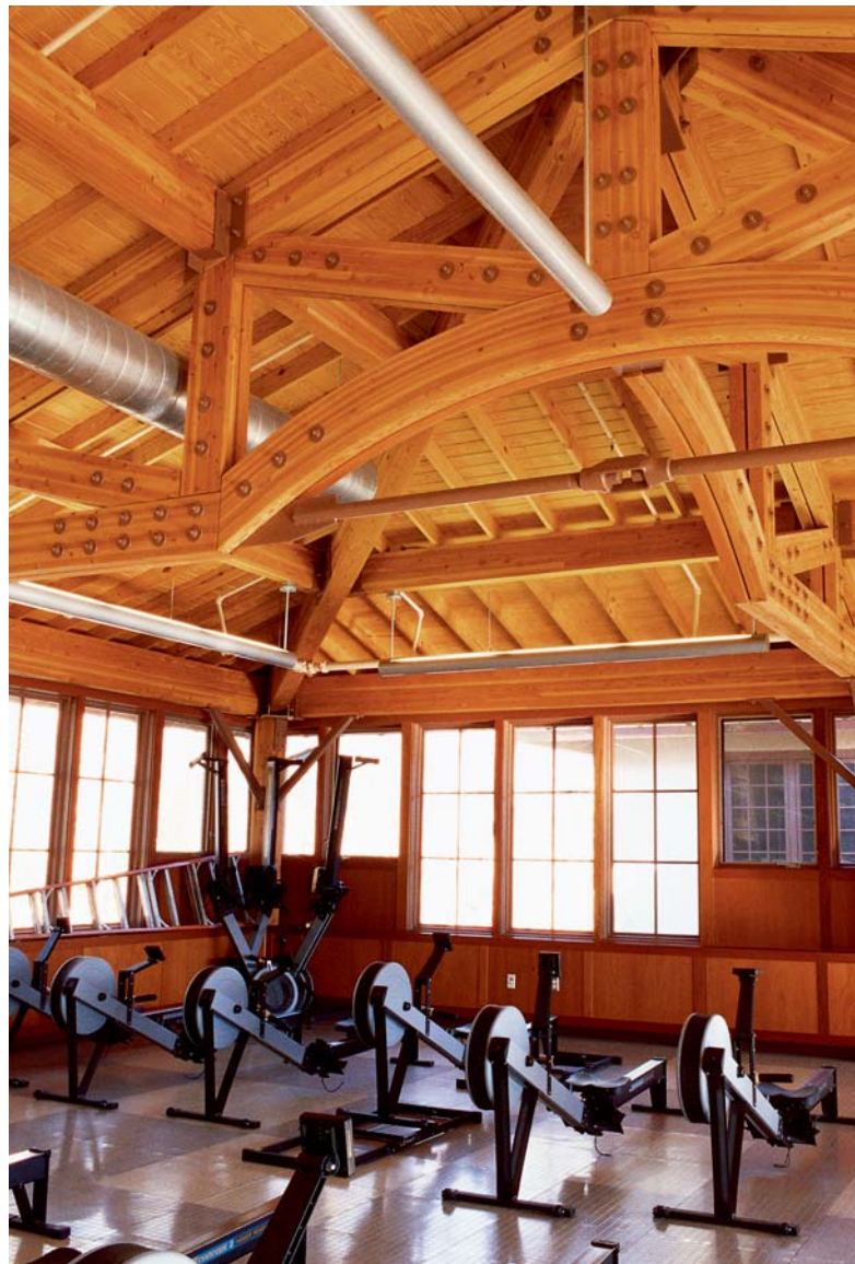
ABOVE: Glulam are a popular choice for the structural systems in recreational spaces. Boathouse, Princeton University.
