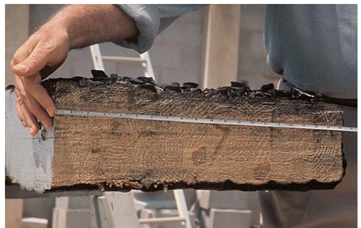
ABOVE (middle): Typical glulam beam enveloped in flames during standard ASTM E-119 fire test.
